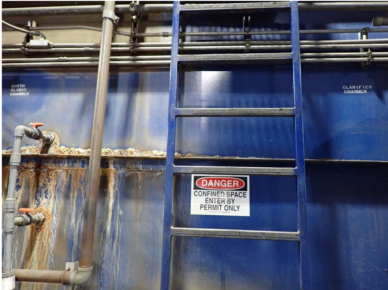
Photo 3: Clarifier chamber and sludge chamber
