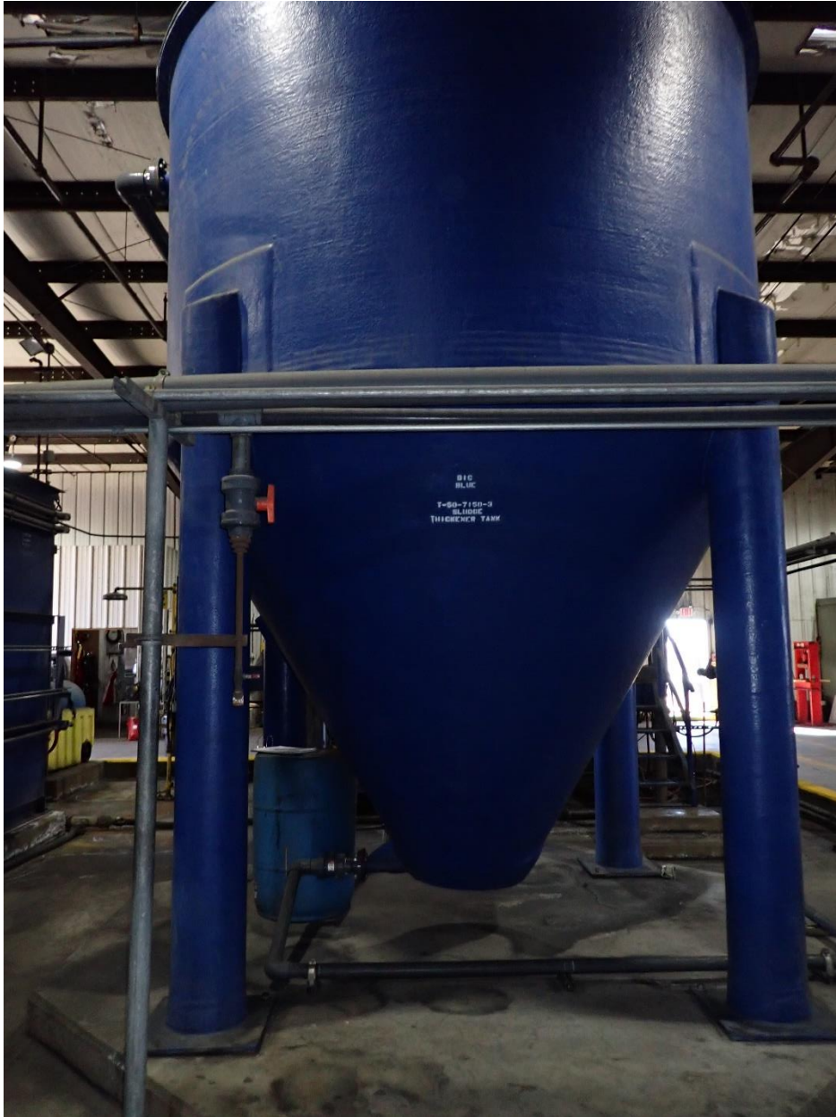
Photo 6: Sludge thickener chamber
