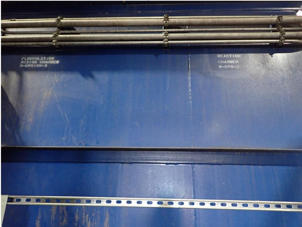
Photo 2: Reaction Chamber and Flocculation Mixing Chamber
