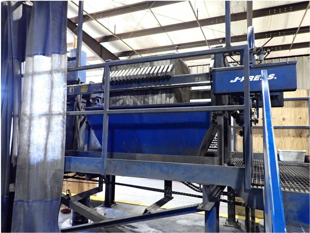
Photo 7: Sludge press condenses sludge into filter cakes, which are sent off-site for disposal.
